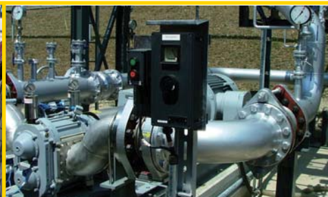
Deloading pump station for biodiesel
